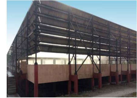
Mist Cooling System
