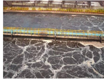
Diffused Aeration System
