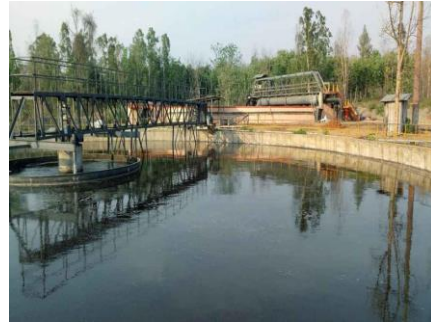
Secondary Clarifier - Pulp
