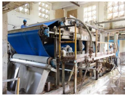
Sludge Handling - Paper
