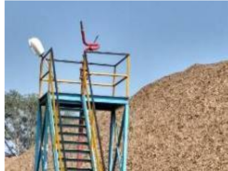
Fire Hydrant Point near chipper
